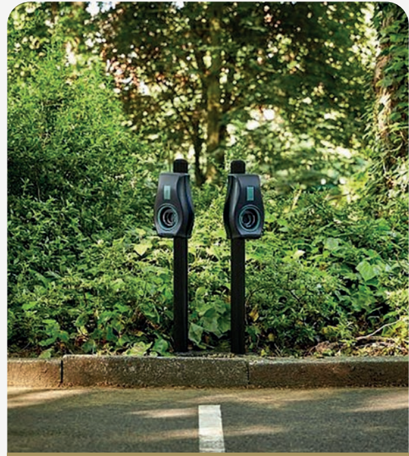
Photo: Connected Kerb bollard charge points in Kent, United Kingdom
